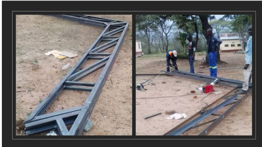
Artisans busy welding the pieces of metal together. When it is all done, they will erect the structure and add roofing using sheet metal.
