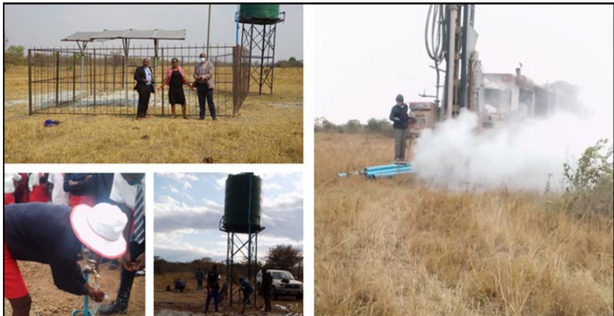
Picture above shows the completed well, the drilling of the well and students testing the water system.
